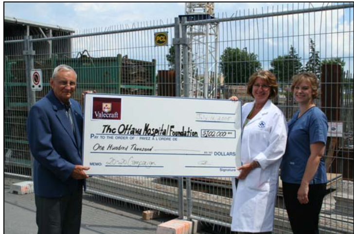
Jean-Guy Rivard of Valecraft Homes presenting a cheque to Joanne Ready and Angela Blasutti (Cancer Centre staff) at the construction site of the expanded Ottawa Hospital Cancer Centre
